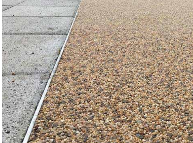
↑ Resin bound gravel to bicycle parking
