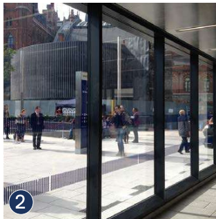
Glazed passenger lift frontage
